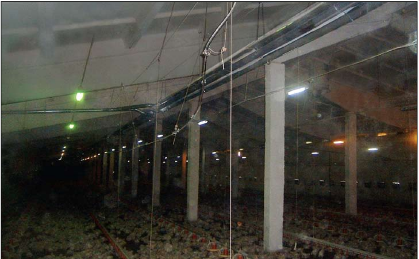
Gas-fired, low-intensity infrared heaters heating a poultry house in Russia.
