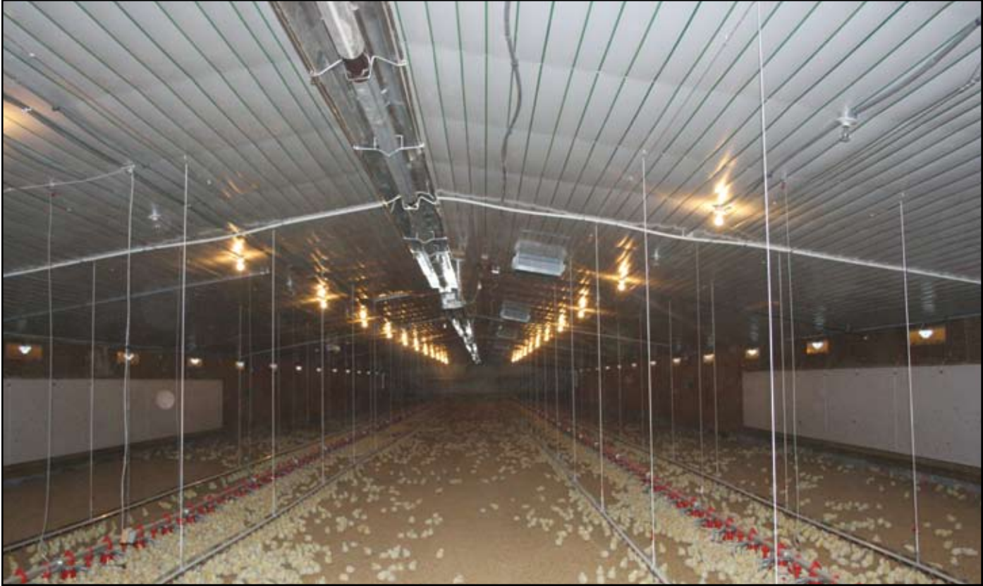
Gas-Fired, Low-Intensity infrared heaters heating a poultry house in the United States.
