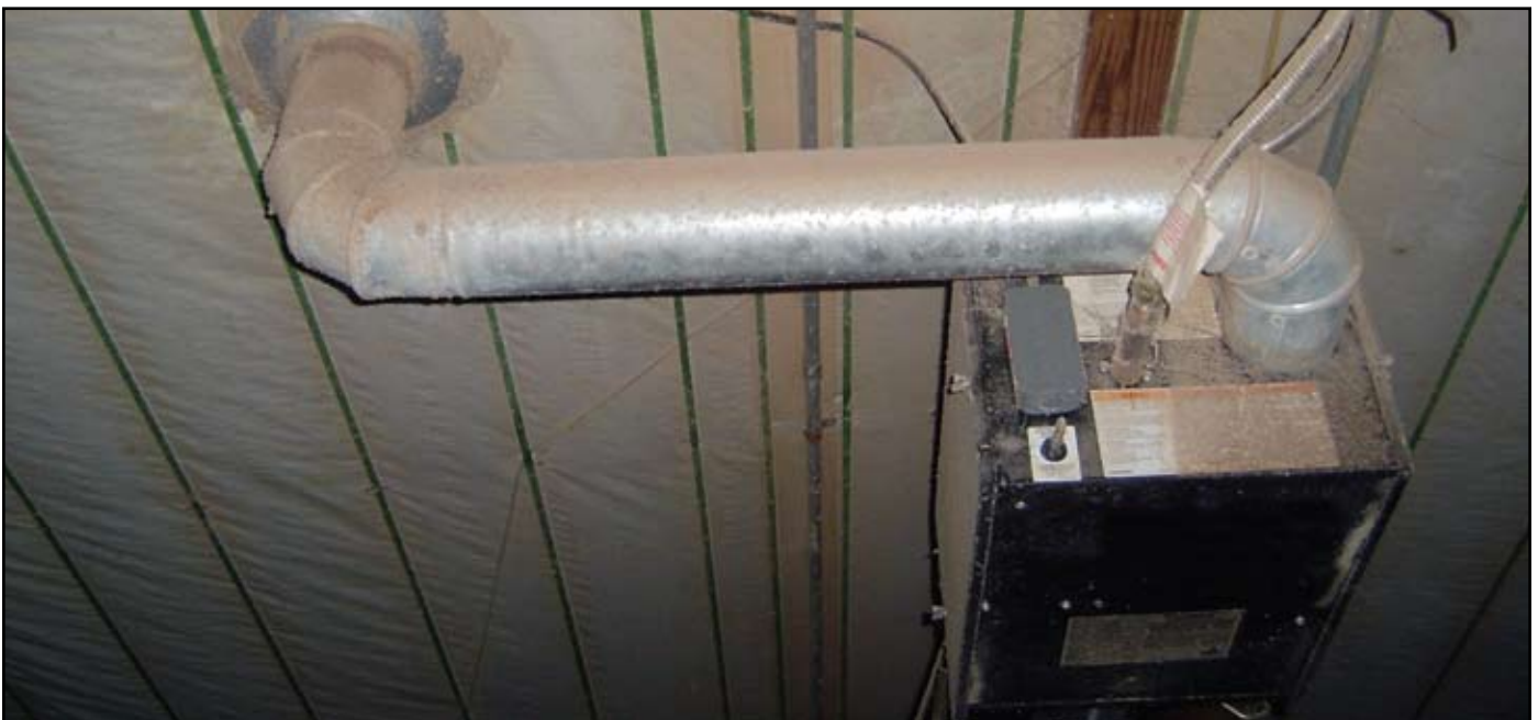
Fresh Air Intake
