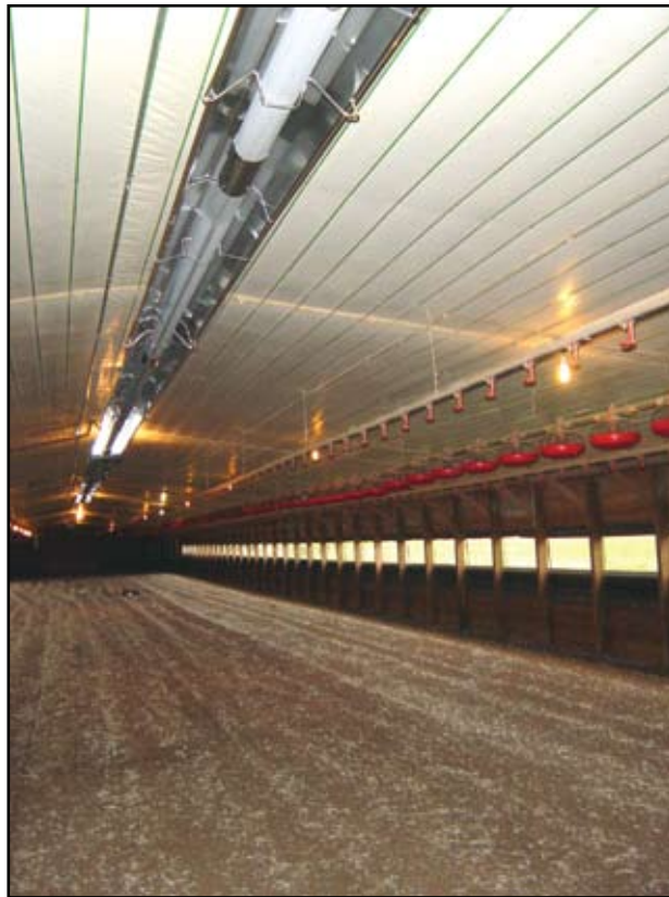
Gas-fired, low-intensity, infrared heaters are overhead and out of the way for house cleaning.
