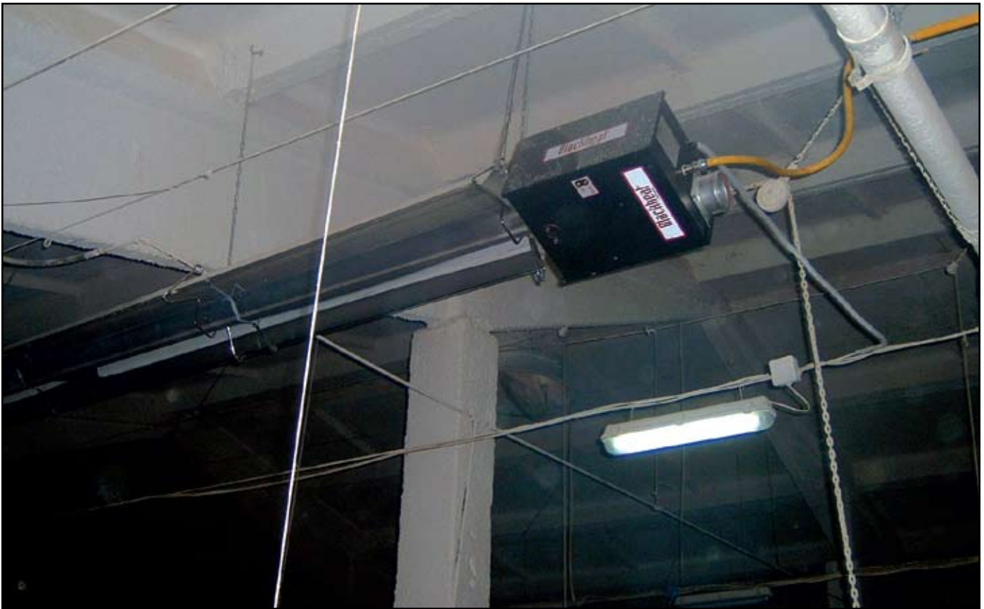
Gas-fired, low-intensity infrared heater being installed in a poultry house in Russia.
