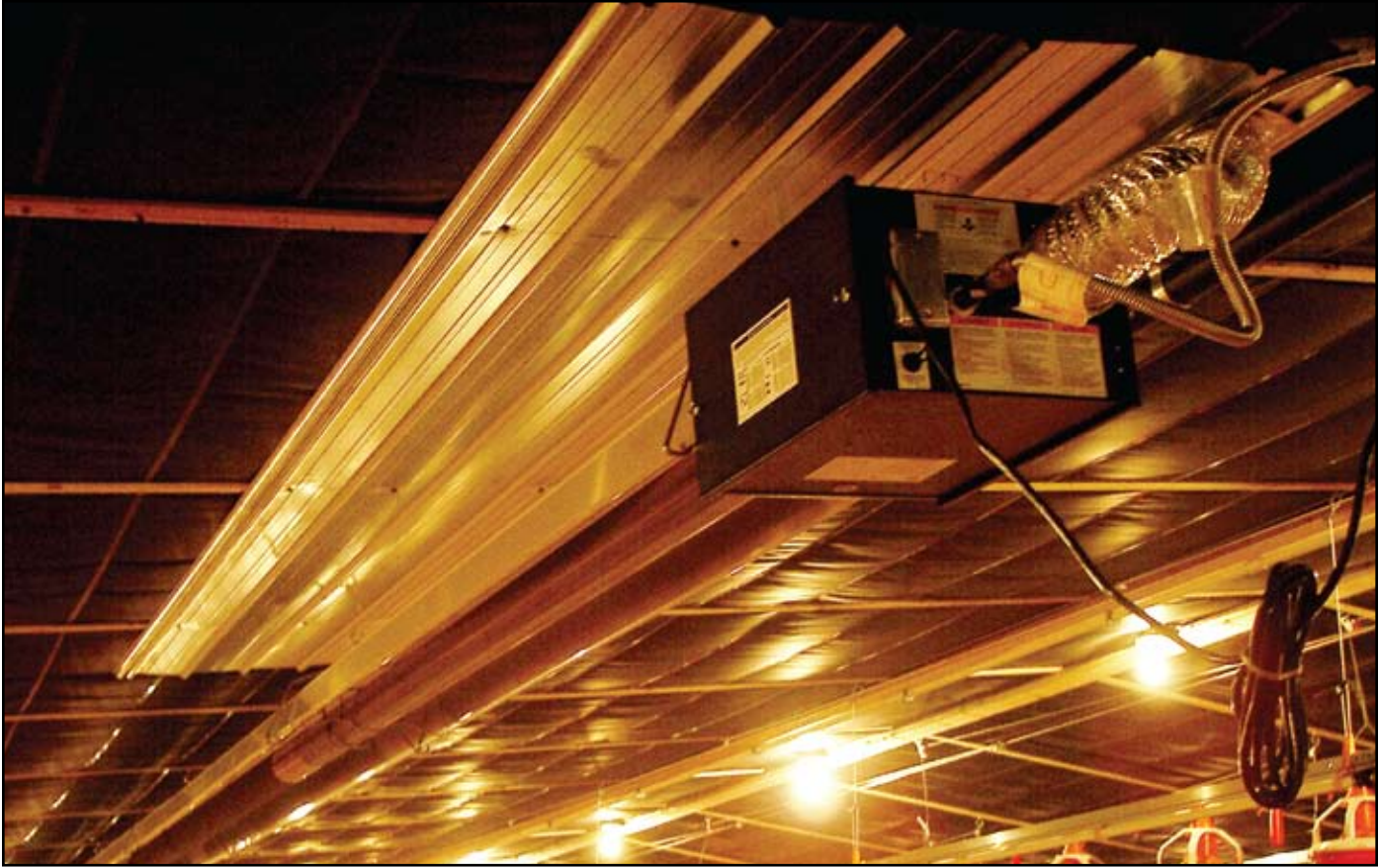
Gas-Fired, Low-Intensity infrared heaters heating a poultry house in the United States.
