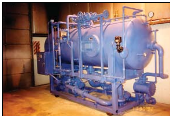
Central Wet System (Boilers)
