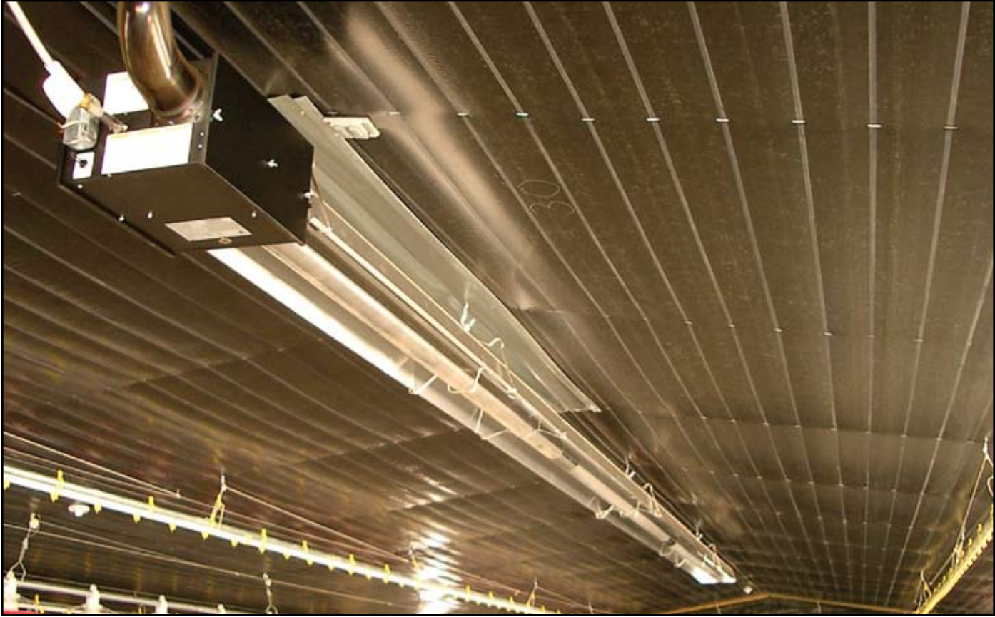
Gas-Fired, Low-Intensity infrared heaters heating a poultry house in the United States.
